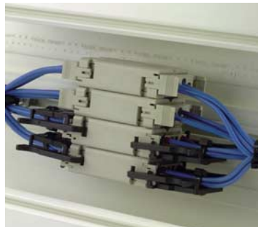
ModuFlex C as coupling in the cable duct
